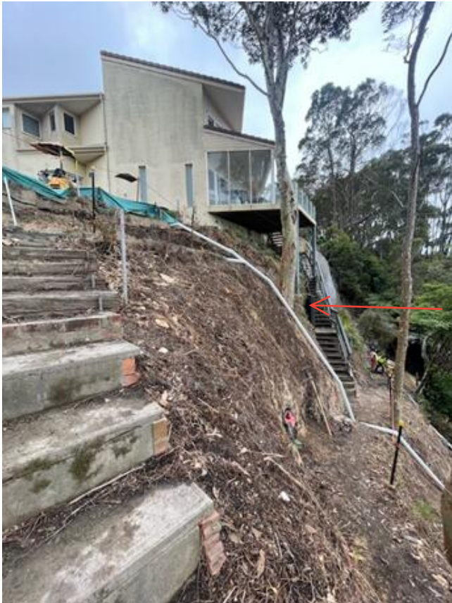
DECEMBER 2023 - PREVIOUS STAIRS AND PATHWAY DESCENDING CLIFF
